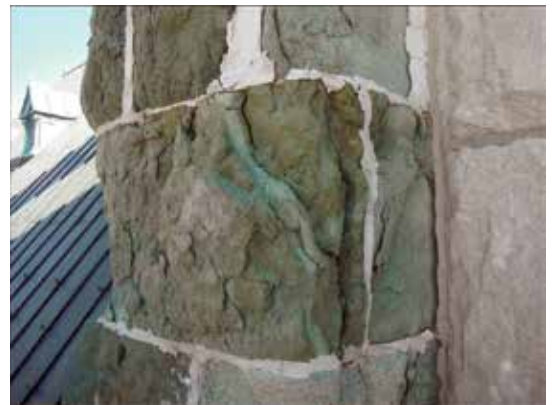
Deterioration of serpentine stone.
